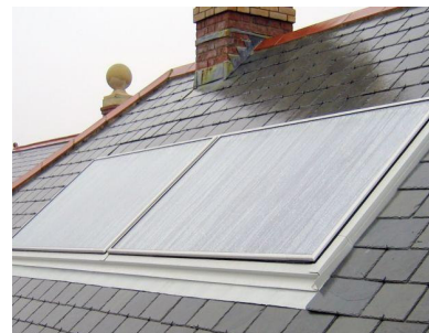
Figure 2: Roof mounted SHW
