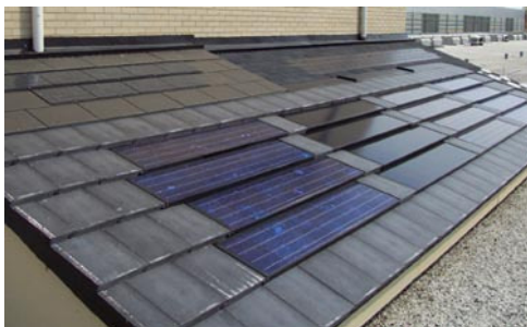
Figure 1: Roof mounted PV
