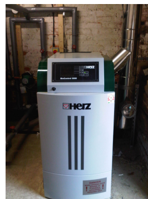
Figure 6: Individual biomass boiler
